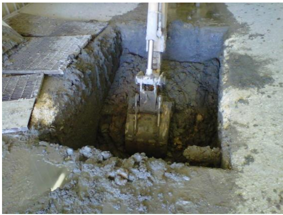
Sump during treatment
